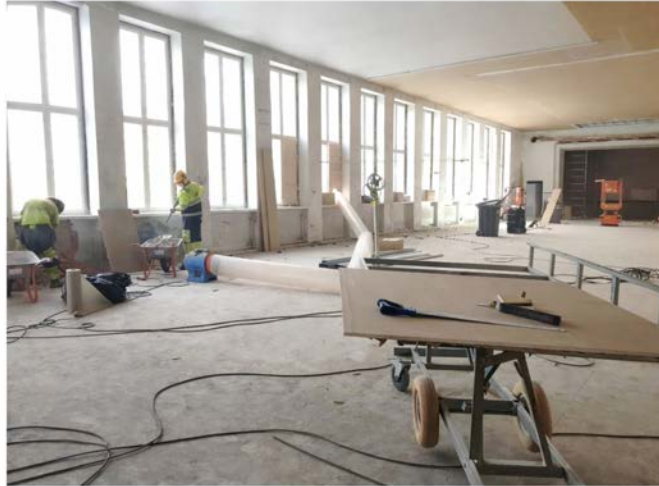
Dust levels cannot be seen with the naked eye, so without measurement there is no way of knowing whether the dust levels at the worksite are within tolerances.
